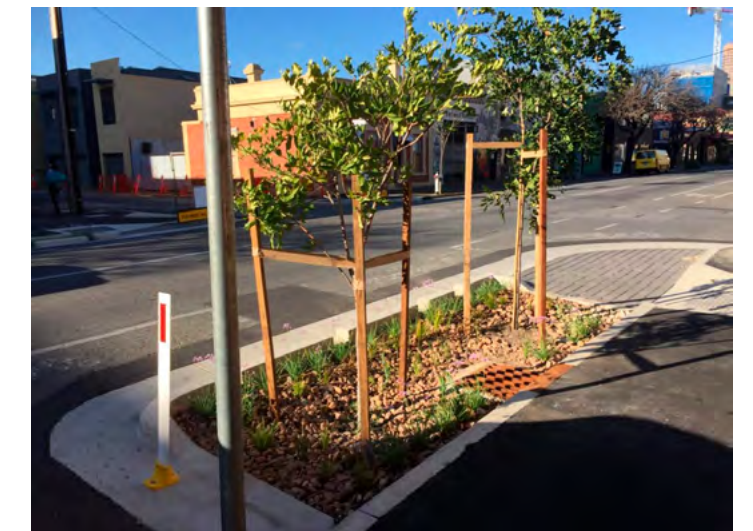
Raingarden/swales including lowered garden area for passive irrigation, and slotted kerbs allowing infiltration from roadway, on Wright Street in Adelaide
