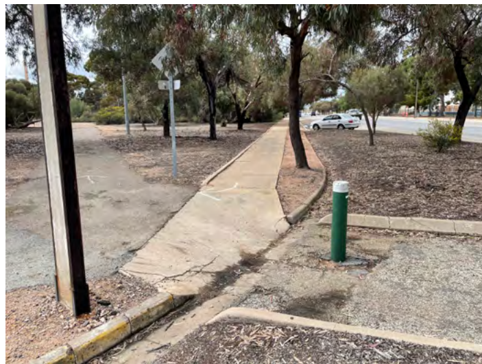
Footpath and ramp in poor condition?
