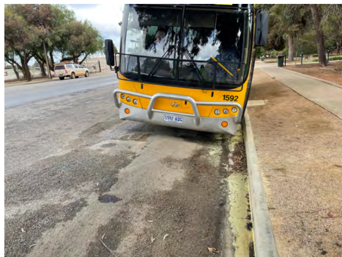
There are issues with water ponding on both sides of the road.
