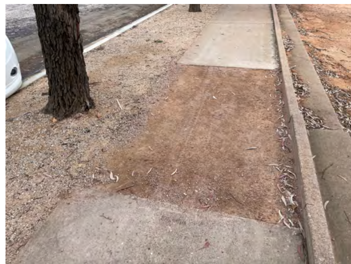
Irregular footpath/kerb on northern side.
