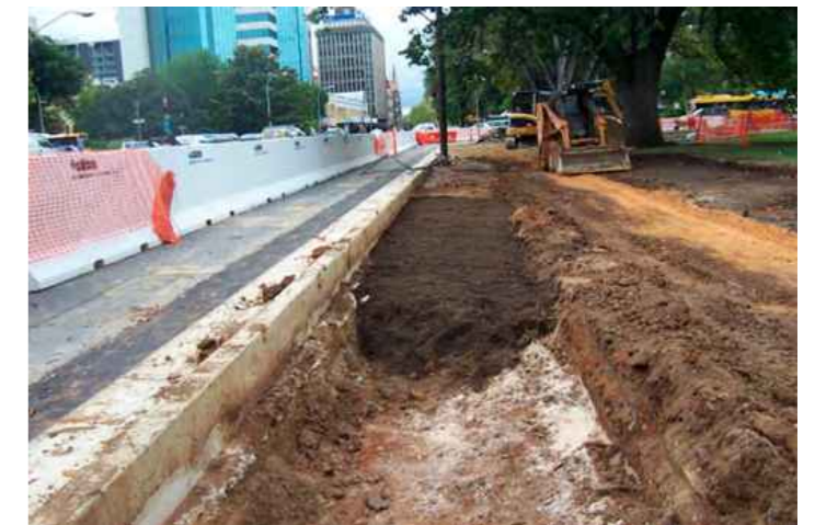
SPACE structural soil with 100% rooting volume being installed on Pulteney Street in Adelaide.
