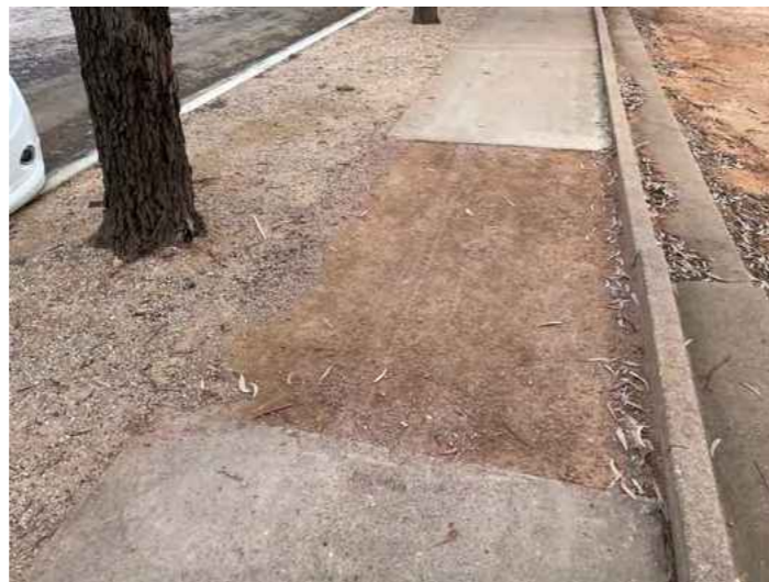
Irregular footpath/kerb on northern side.
