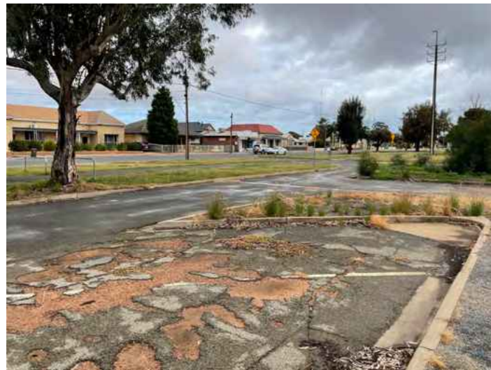
The western entrance of the park has a disorderly roadway, lacks pedestrian sidewalks, has poor visibility, and suffers from severe road surface damage.
