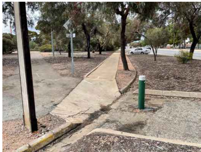
Footpath and ramp in poor condition?
