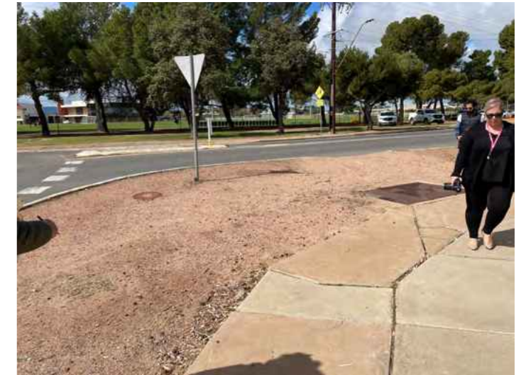
There is no vegetation cover around the roundabout, and the crossing is not connected to the footpath.
