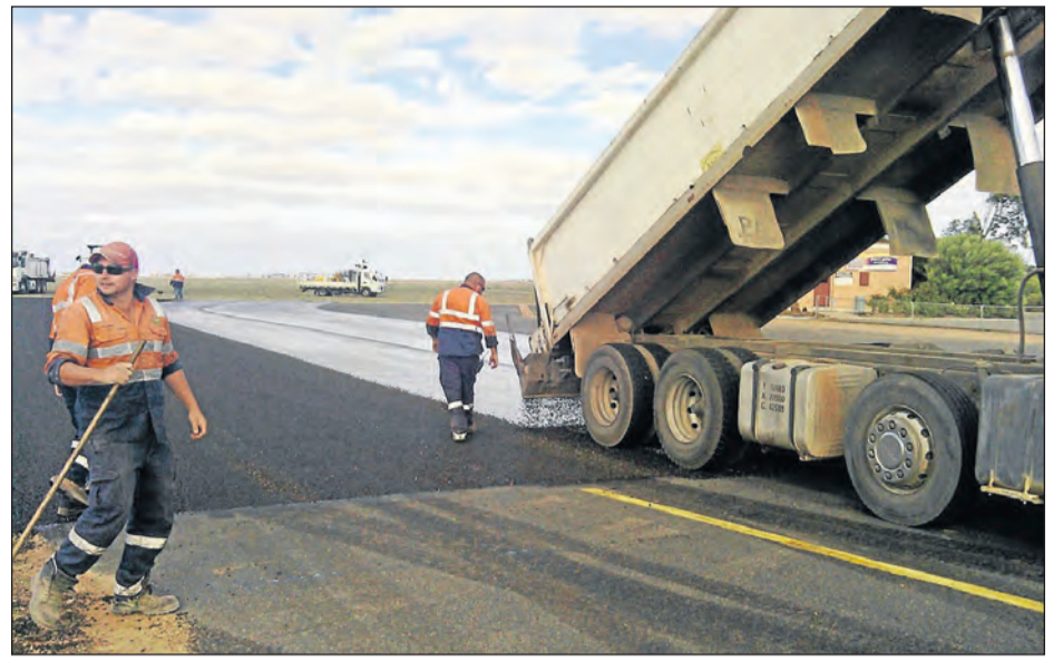
RESEALING... Port Pirie Regional Council resealed sections of road at the Port Pirie Aerodrome in February, 2015. This photo demonstrates the resealing process which will be carried out on approximately 23 kilometres of road in 2015/16.
