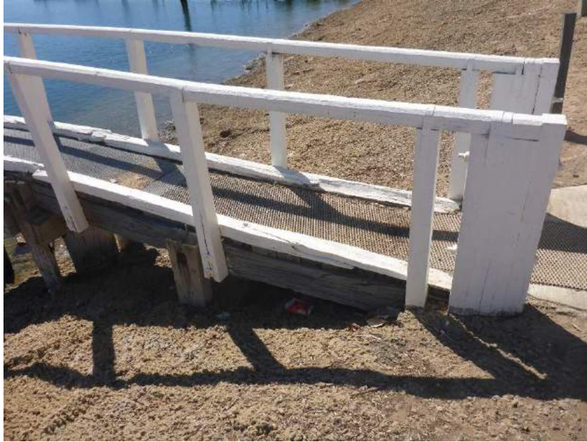
Photo 4 – Jetty abutment with large vertical timbers at the end of the handrail
