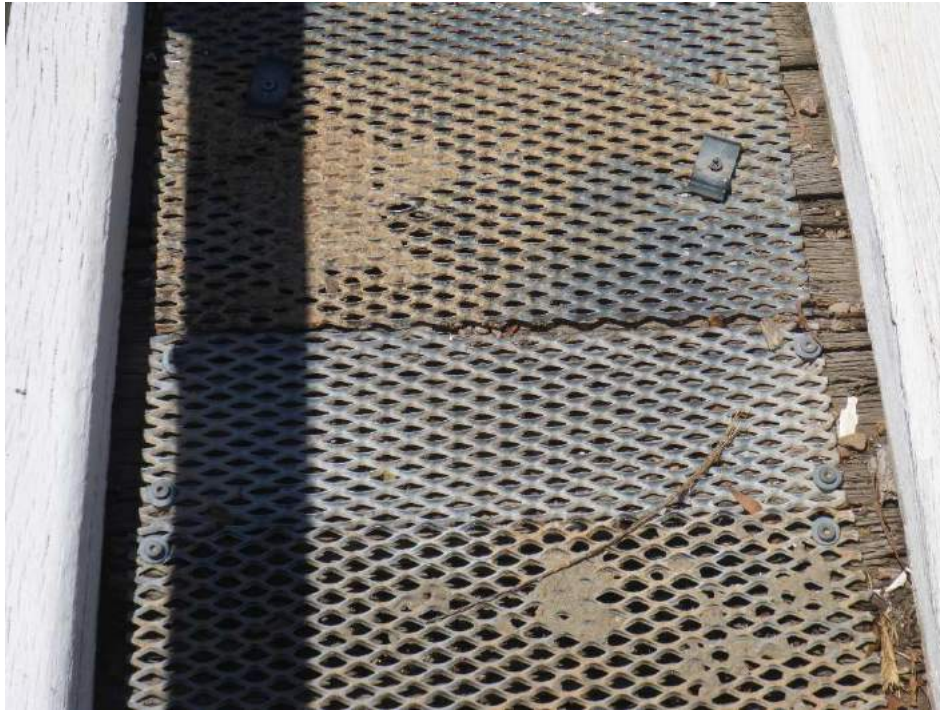
Photo 6 – Weathered and loose timber planks
