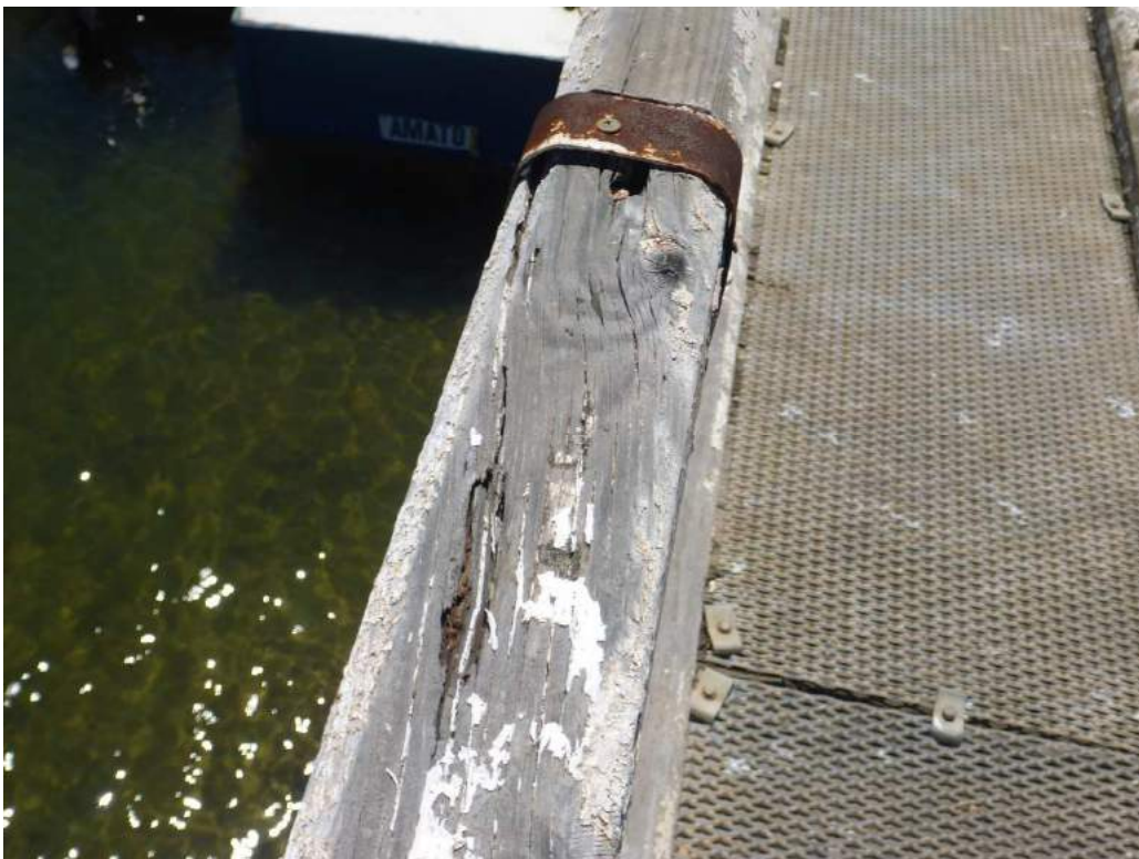
Photo 12 – Section of cracked and rotted top rail with rusted steel strap
