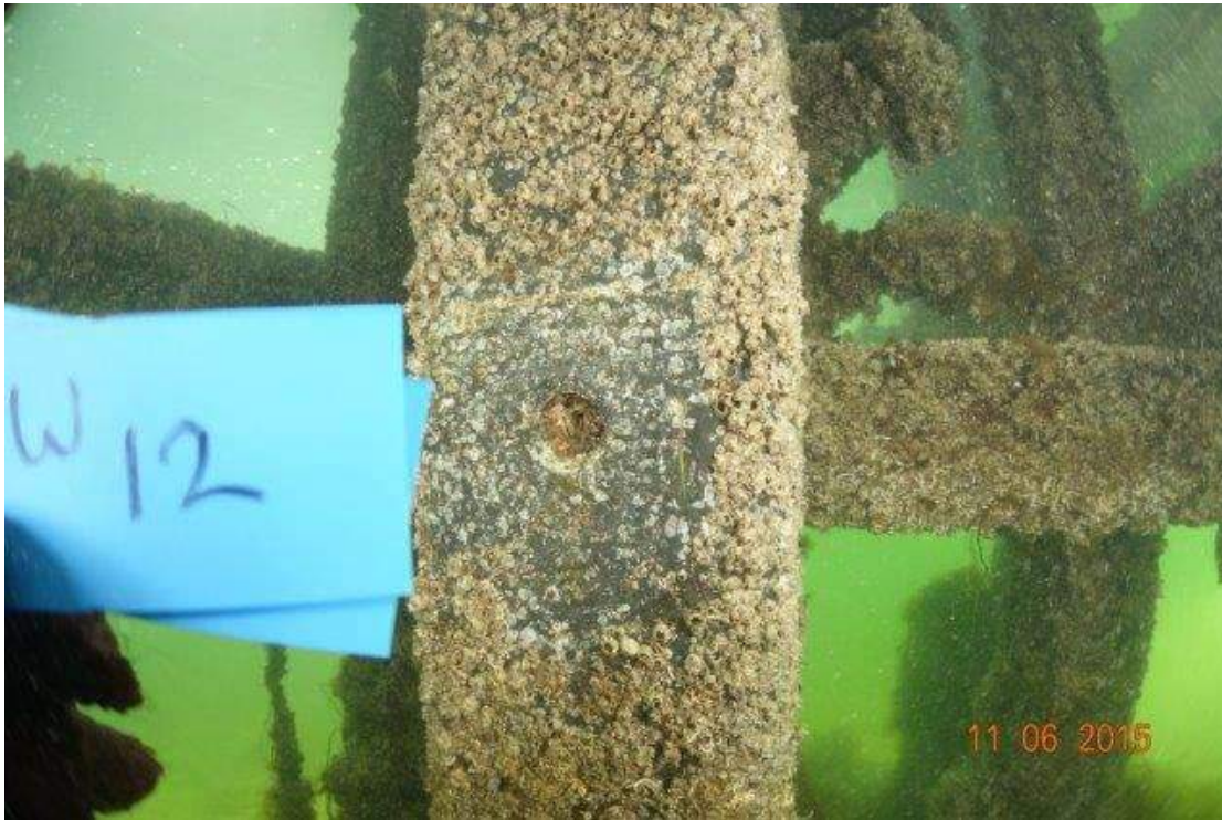
No bolt fitted at pile 12
