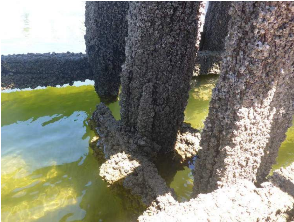
Photo 18 – Badly deteriorated timber bracing
