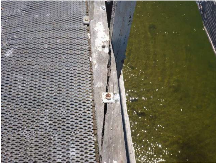
Photo 8 – Section of badly cracked kickboard
