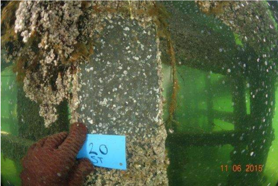
Typical condition of steel pile where cleaned of marine growth (paintwork intact, no signs of corrosion)
