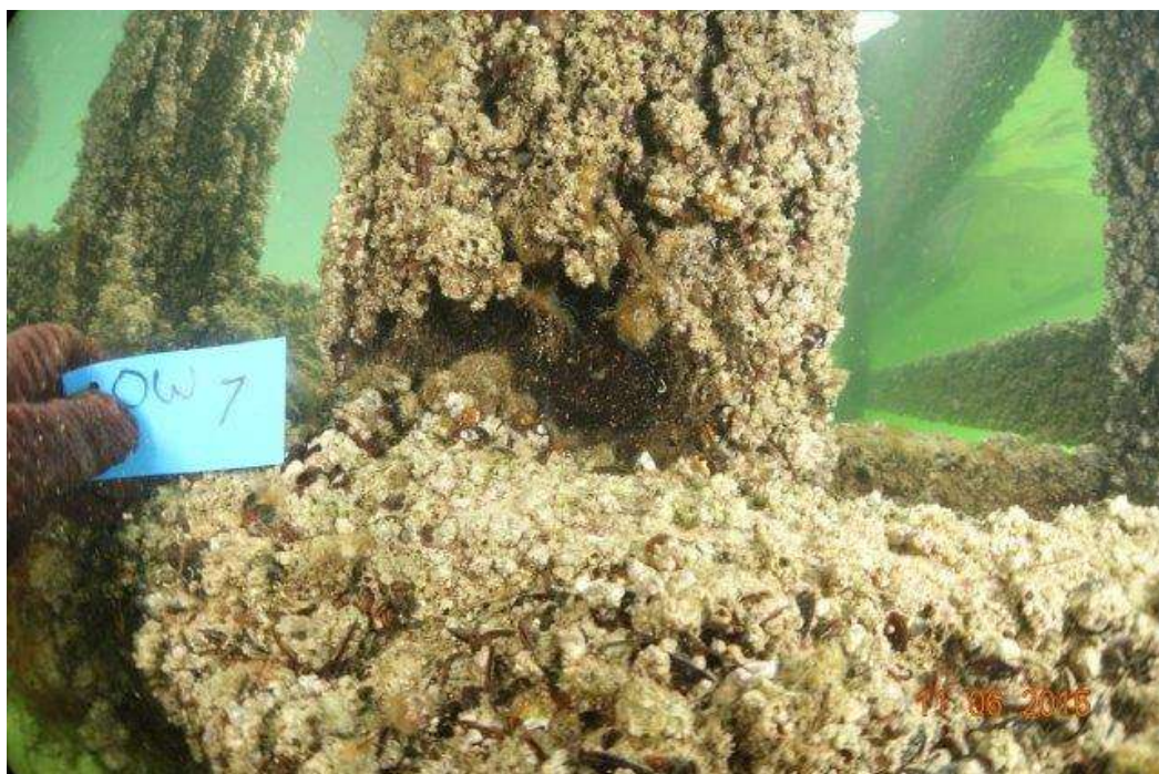
Bent 7 outer walkway pile defect at the crosshead
