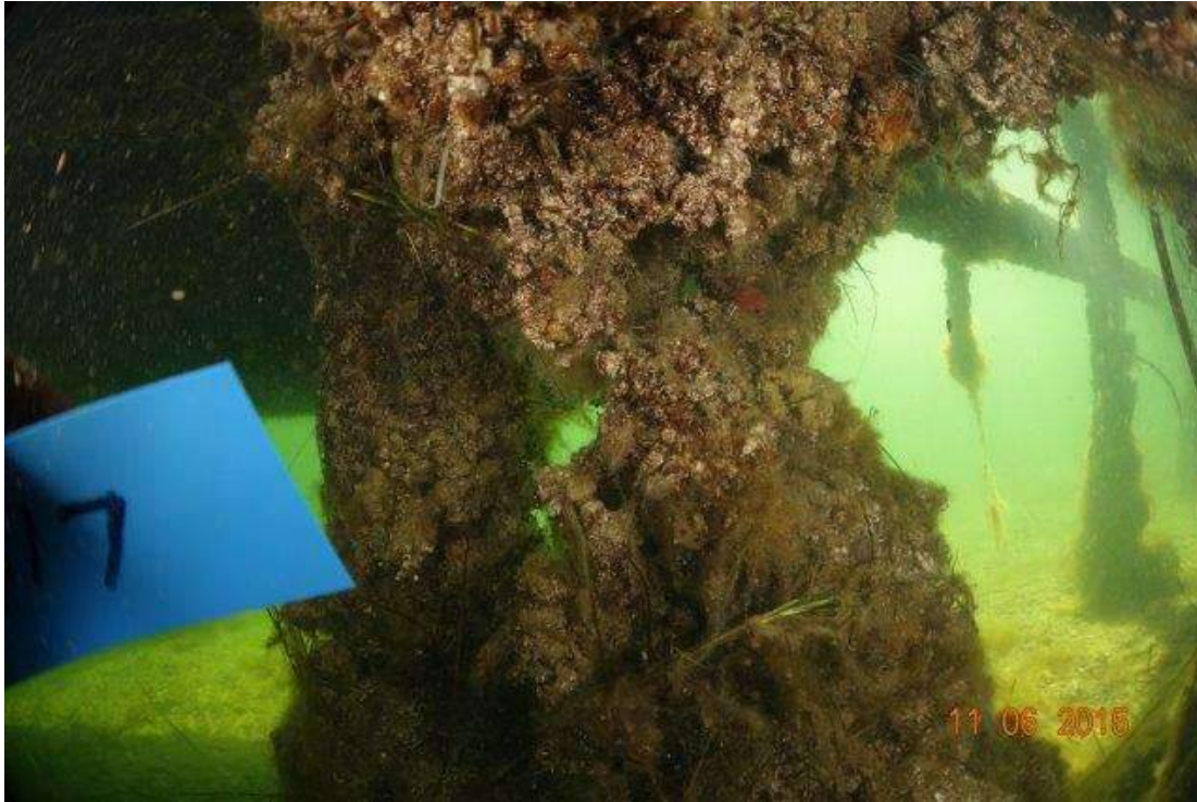
Photo illustrates pile at bent 17 fully deteriorated
