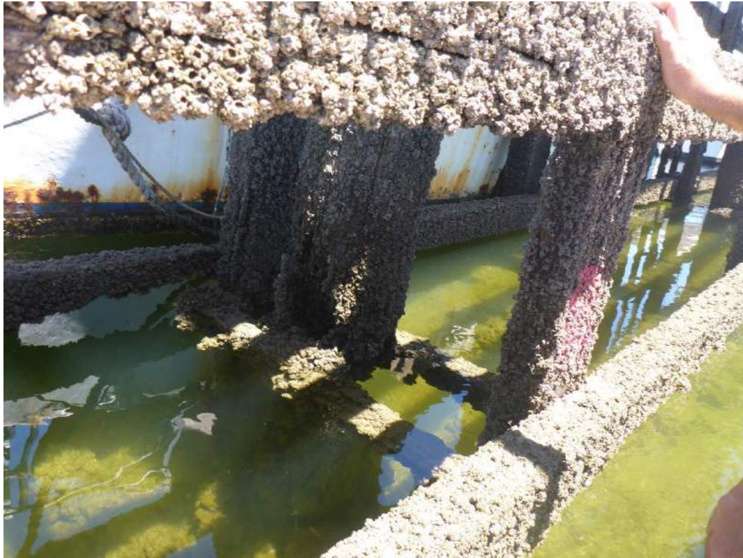
Photo 23 – Badly deteriorated pile but difficult to determine extent of deterioration without underwater assessment
