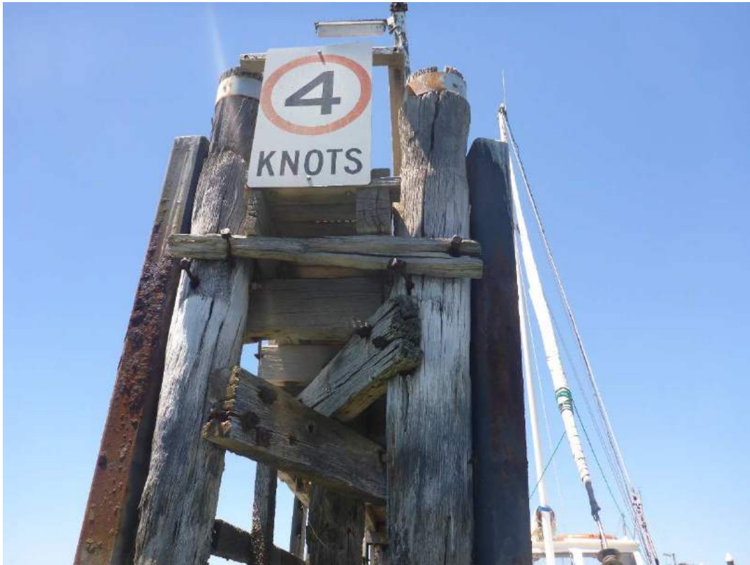
Photo 22 – Two steel piles at the end of the outer walkway with quite heavy corrosion
