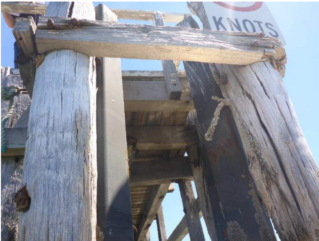
Photo 21 – Two steel piles at the end of the main walkway showing some corrosion
