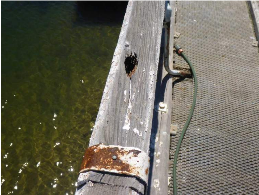
Photo 11 – Section of rotted top rail and rusted steel strap
