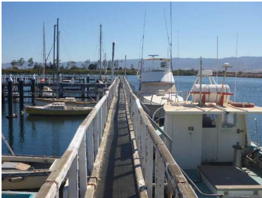
Photo 9 – Handrails both sides with poor shape and alignment
