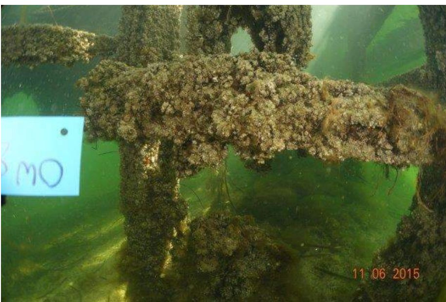
Outer walkway bent 8 illustrating fully broken pile
