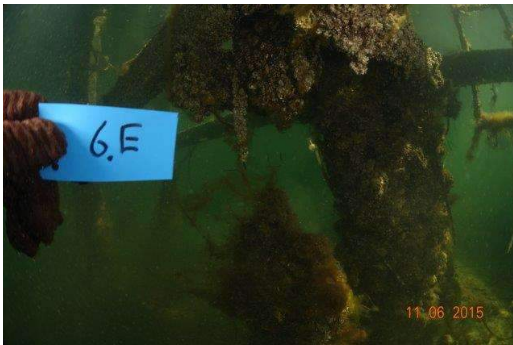
Photo illustrates broken vertical rectangular timber fender adjacent to pile 6 on the eastern side
