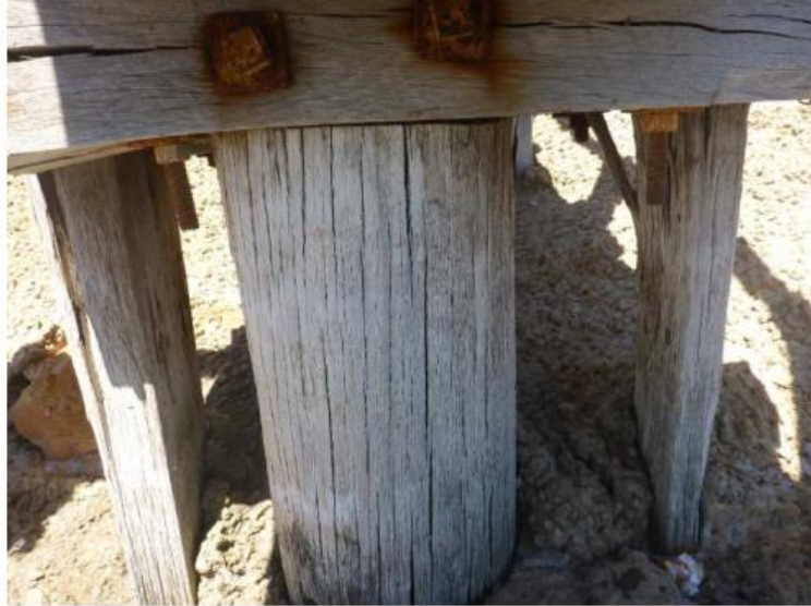
Photo 19 – Typical main set of pile layout with a central circular pile and two rectangular piles
